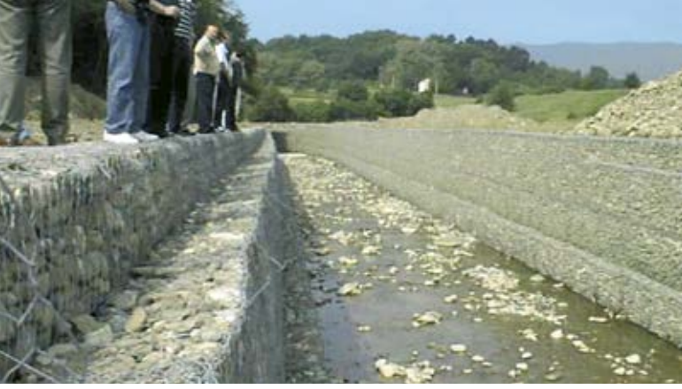
Figure 3 ► Vertical gravitational revetment made of gabion mattresses
